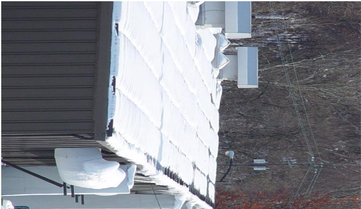
Typical heat loss associated with inferior insulation tactics such as vinyl faced fiberglass batt's installed during construction of pre-engineered buildings.
